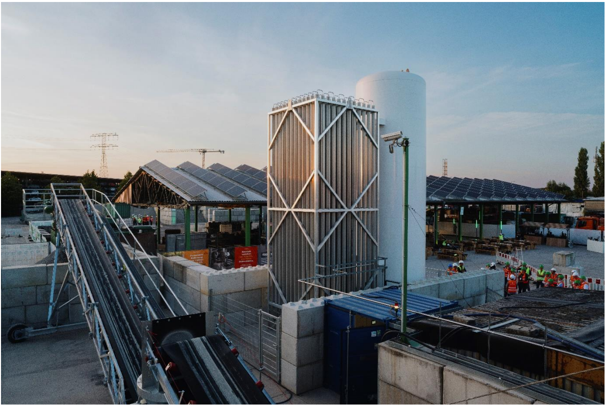
Figure 2 – A neustark CO 2 storage plant operating in Berlin, Germany, with a capacity to remove 1000 tons of CO 2 per year.
